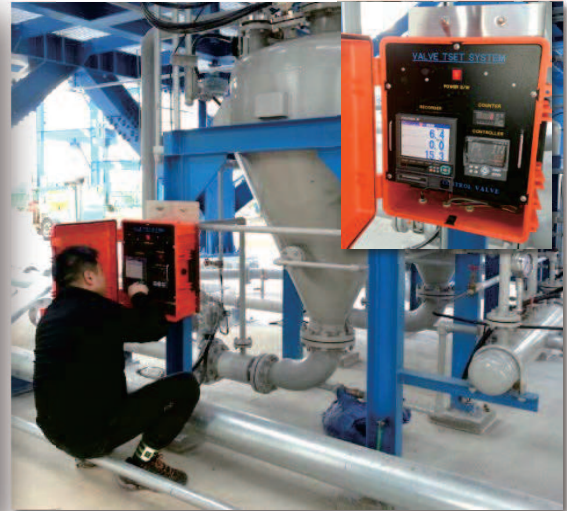
The installed valve recorder at the field to check the status and lifespan of valve .
